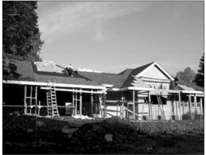
Gateway residents are eagerly awaiting the completion of the new Gateway Manor. In the fall, the Residential Department looks forward to inviting all to an open house.
